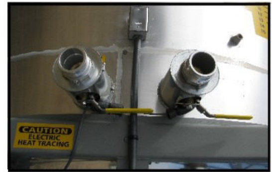
Insulated ball valves at the base of the tank gravity feed emulsion to the Total Patcher.
