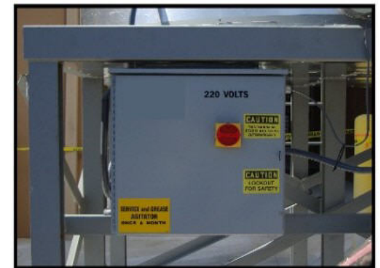
Electrical control panel and agitator timer is enclosed within a single weatherproof NEMA 3R enclosure.
